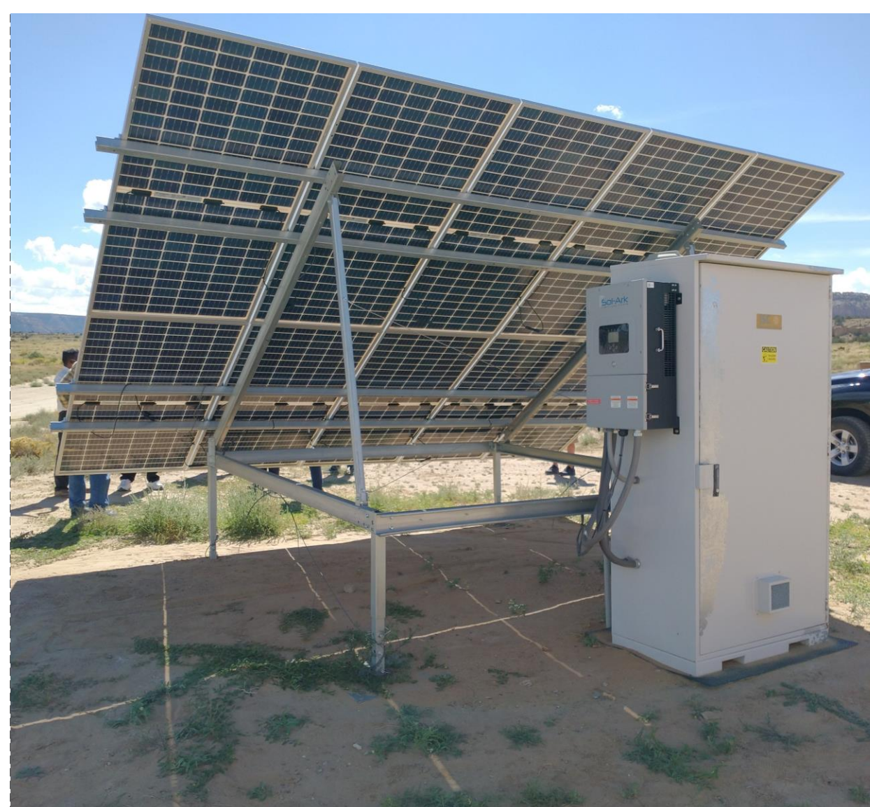
Fig. 2: An off-grid solar system with 3.8 kW bi-facial array, 35.1 kWh gel battery bank and 8 kW inverter.
